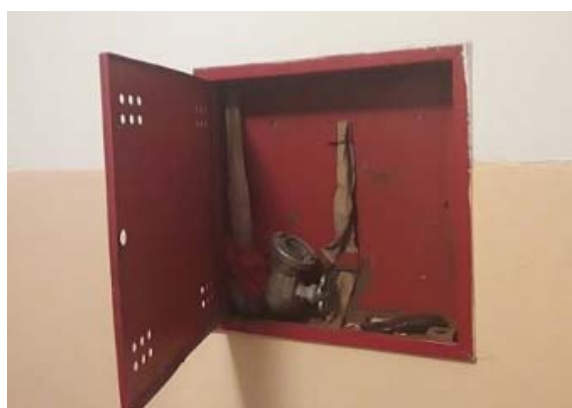
Damaged and unusable hydrant
