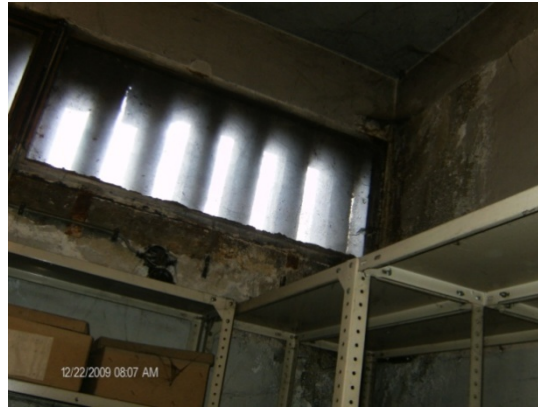
Water leakage in the depot
