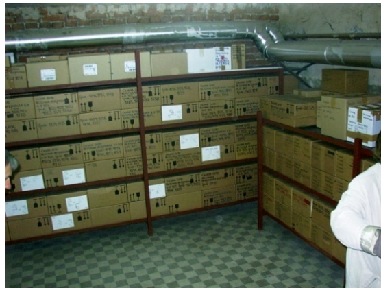
Pipes of central heating
