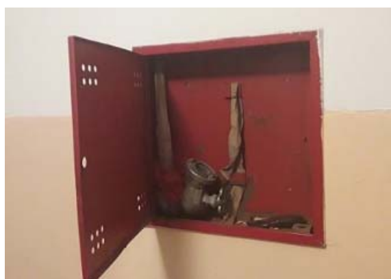
Damaged and unusable hydrant
